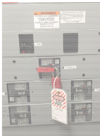
Breaker Box lock
